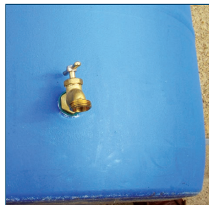
Figure 17. Hose bib facing down.
